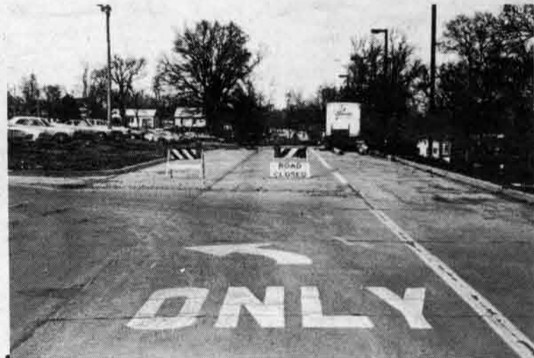
The nearly completed East Drive, a familiar sight to UMSL-ites. photo by Steve Kator
